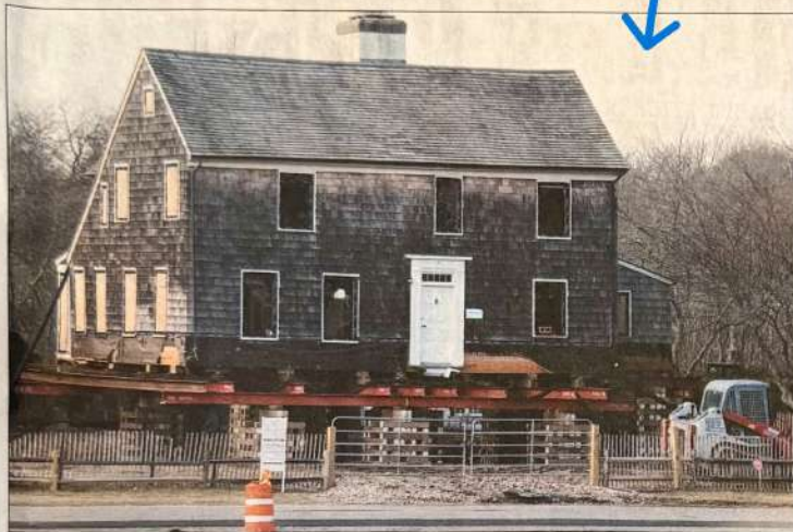
How do you lift a house that's almost 300 years old? Very, very carefully.
